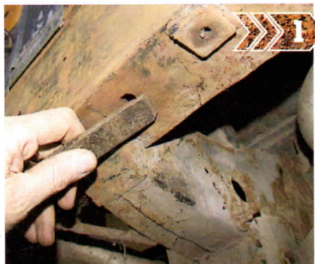
Scrape away loose rust and paint, then use a wire brush. Manufactured holes in the chassis will be handy for injecting wax
