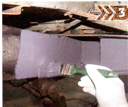
After rust converter, a coat of rust-resisting primer provides a base for a final layer of your preferred top coat
