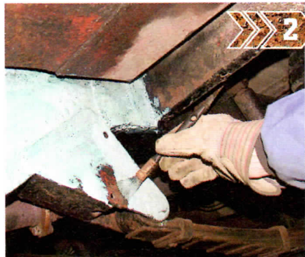
Now apply rust converter. Neutra Rust converts surface into corrosion-resistant barrier and dries to a dark colour
