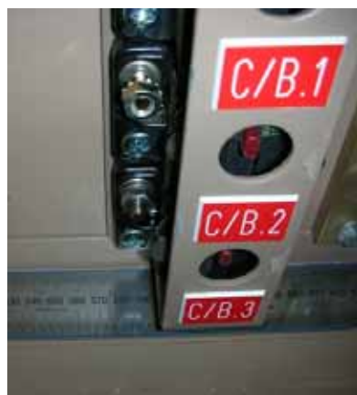
Figure 29 Mounting of the 24-volt Auxiliary Load Centre Circuit Breakers
