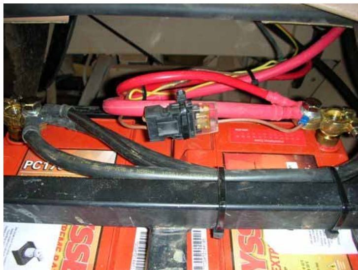
Figure 49 Alternative View of the Left-hand Battery Bank Installation
