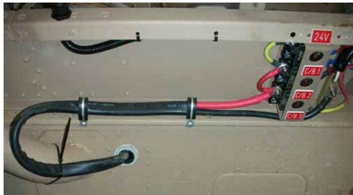
Figure 47 Cable Route Along the Underside of the Combing
