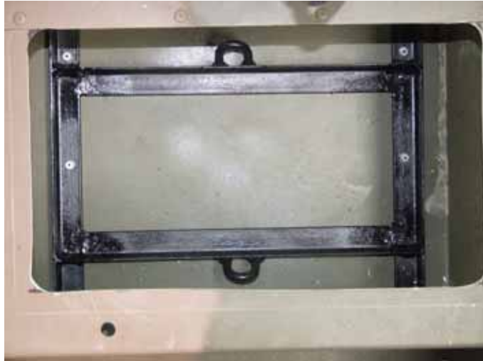
Figure 14 Battery Box Opening Showing Battery Mounting Frame in Position
